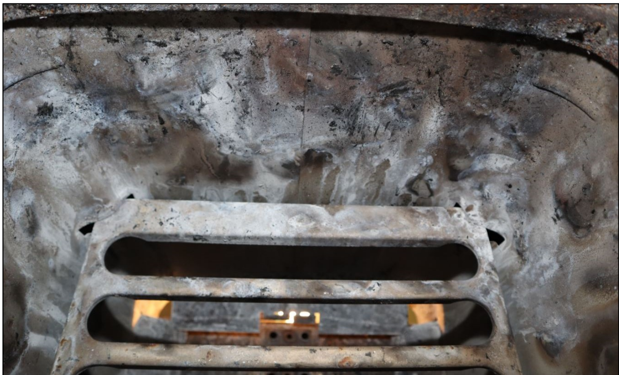
Figure 12. There were bulges of different sizes throughout the heater's stone space casing. The heating elements were not in place when the photos were taken.
