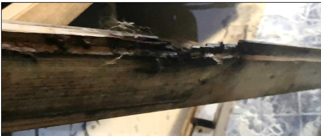
Figure 20. In the Päijät-Häme fire, the wall panel behind the sauna heater was significantly charred. (Photo: Päijät-Häme Rescue Department)
