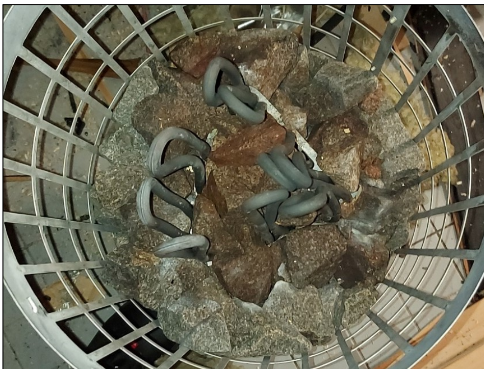
Figure 21. When stones were removed from the heater involved in the fire in Kanta-Häme, it was found out that they were compacted to a significant degree. Heating elements of the heater were bent so that some of them were touching one another. The stones in the middle of the heater were discoloured. (Photo: Kanta-Häme Rescue Department)
