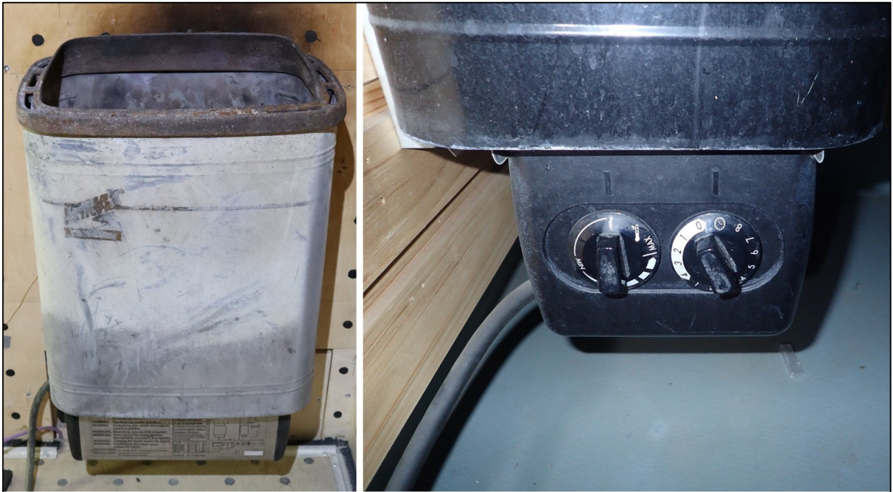
Figure 6. In the photo on the left, the burnt heater after it was re-electrified and on the right the controls of another heater of the same age. The heater in the photo on the right is in the sauna of another apartment in the same building. (Photo: Safety Investigation Authority, Finland)
