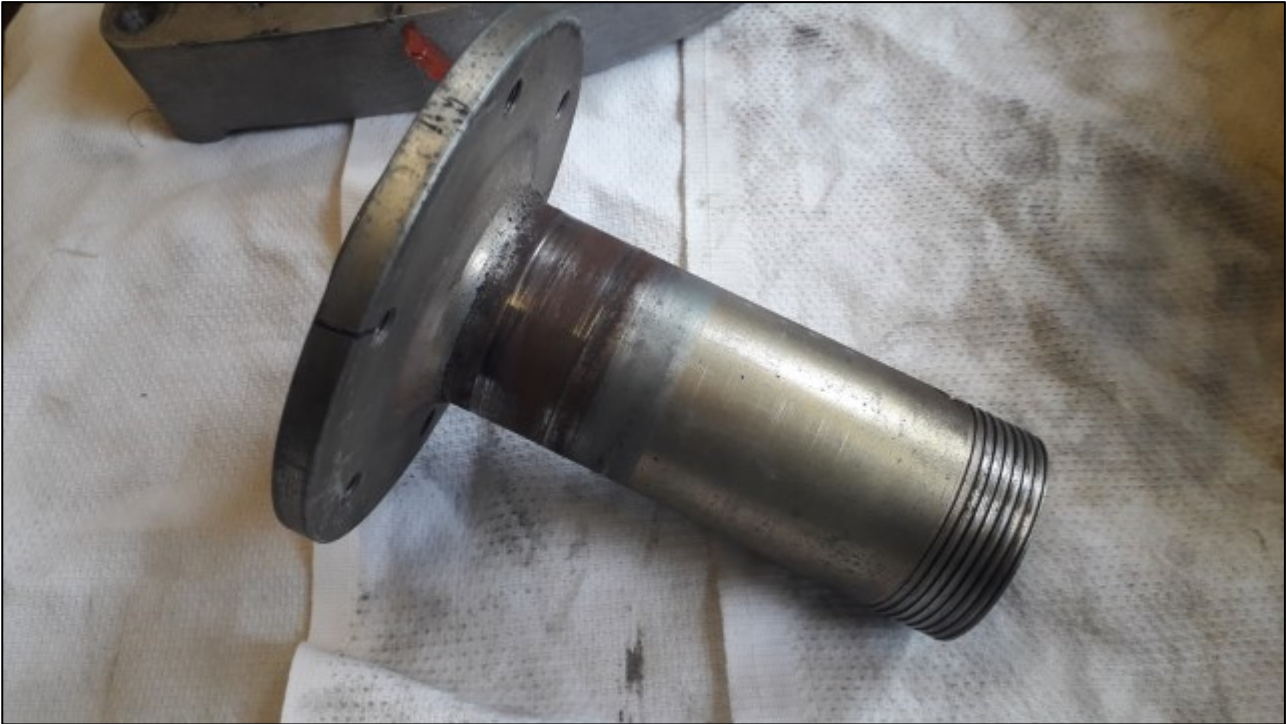
Figure 11. The propeller shaft and propeller mounting flange. Abrasion caused by the contact with the bearing and dust corrosion are apparent around the left-hand end of the shaft. (Photo: SIAF)
