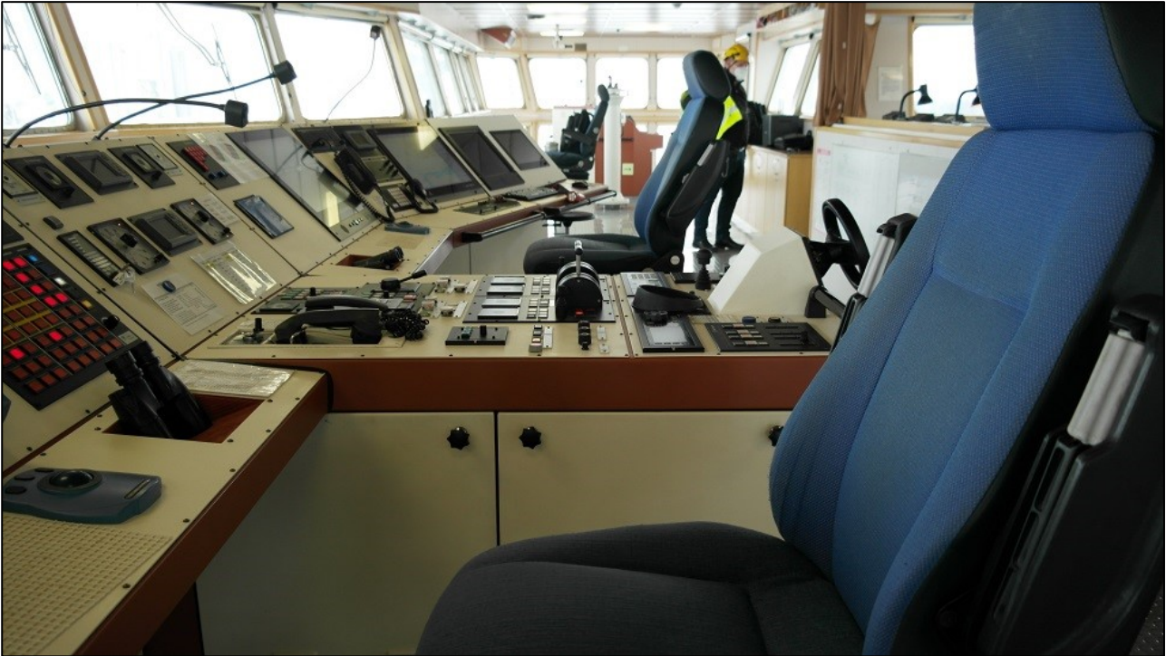
Picture 7. Workstations on the bridge, with a helm in the central console for manual steering. (Image: SIA)
