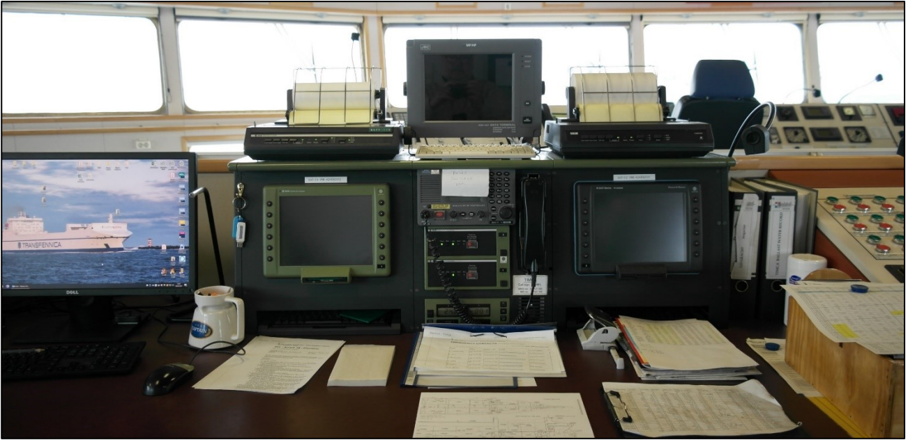
Picture 11. The vessel's GMDSS radio station. (Image: SIA)
