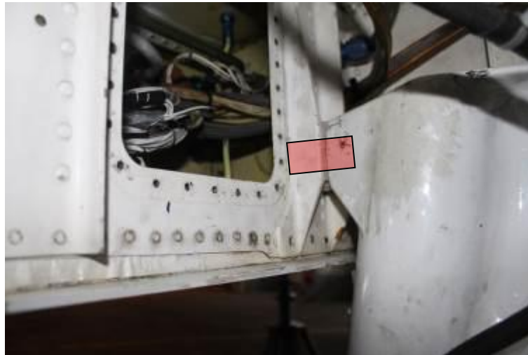
Kuva 3. Forward attachment point of the right main landing gear in place. The location of the pivot pin is shown by a red rectangle. The pivot pin is removed and fitted through an open access panel. Picture: Lapin Tilauslento Oy
