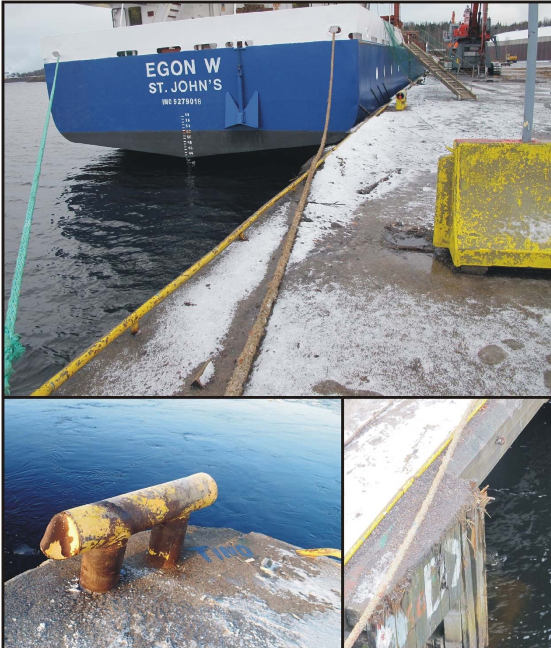
Figure 15. On the day following the accident, wooden waste increasing risks related to moving and working on the quay could be observed on edge parts of the quay top (topmost photo). There was also an end flange which was torn from the joint and twisted at the mooring bollard at the corner of the quay as well as splinters of wood in the protective balks on the quay. Both these factors may have made line handling more difficult. (photos: the police, the SIAF)
