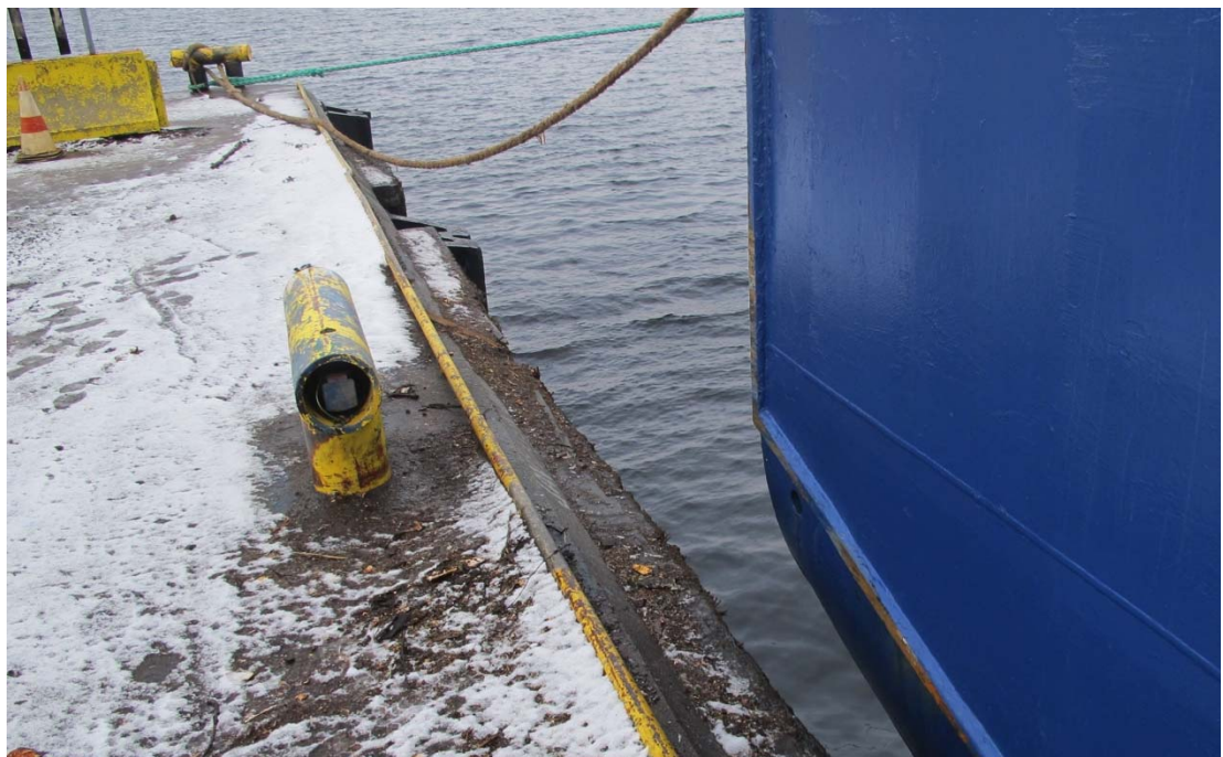
Figure 4. The concrete quay top at the scene of the accident, at the west end of quay B. An edge block made of yellow metal tube, the starboard side stern corner of the EGON W and the wooden protective beams on the edge of the quay can be seen in the photo. Photo taken on 27.11.2013. (photo: the police)
