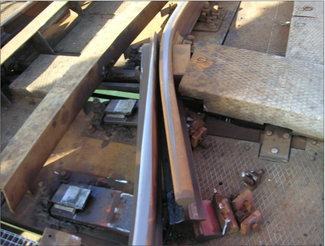
Figure 15: Collision Damage to the Railway Bridge Source: DMAIB
