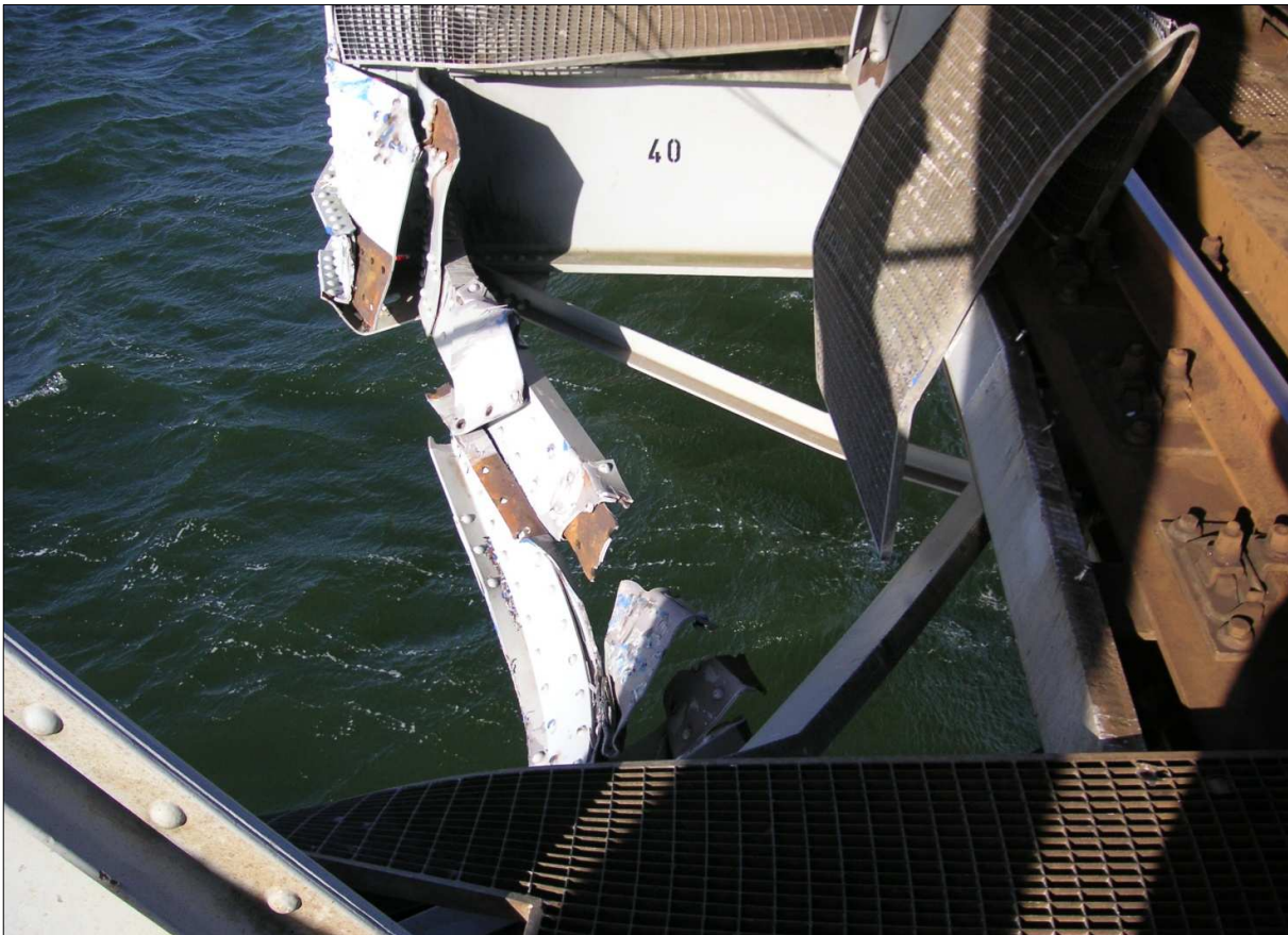
Figure 13: Collision damage to the Railway Bridge Source: DMAIB
