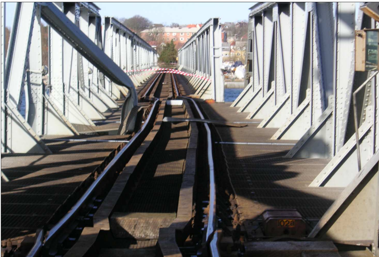
Figure 14: Collision Damage to the Railway Bridge Source: DMAIB
