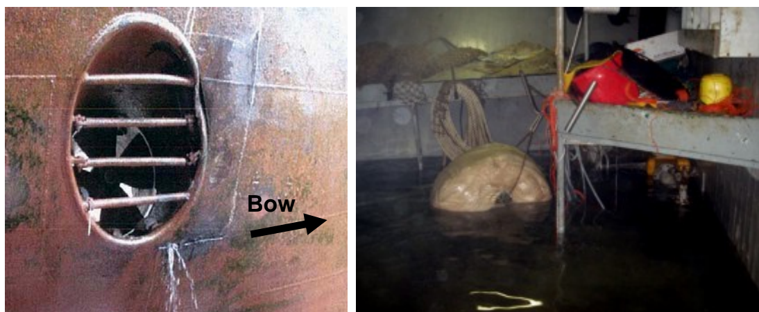
Figure 11. Left: damage on the starboard side of WILLEMPJE HOEKSTRA, in the bow thruster tunnel.
