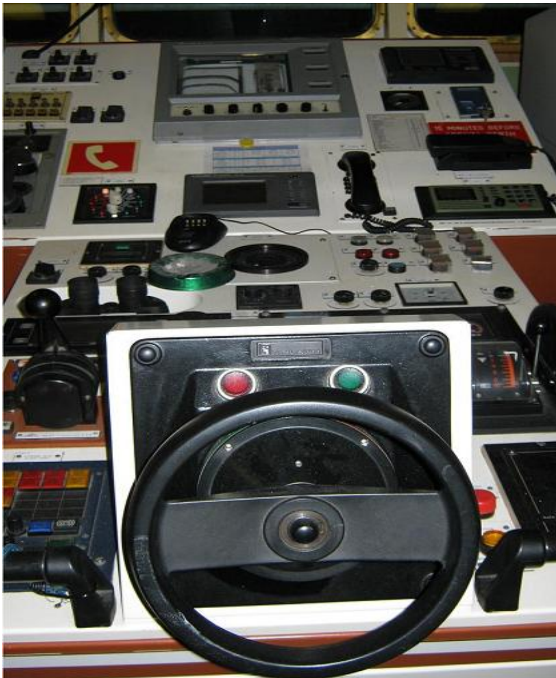
Figure 3. General arrangement of the bridge, control devices and steering stand in the middle console.
