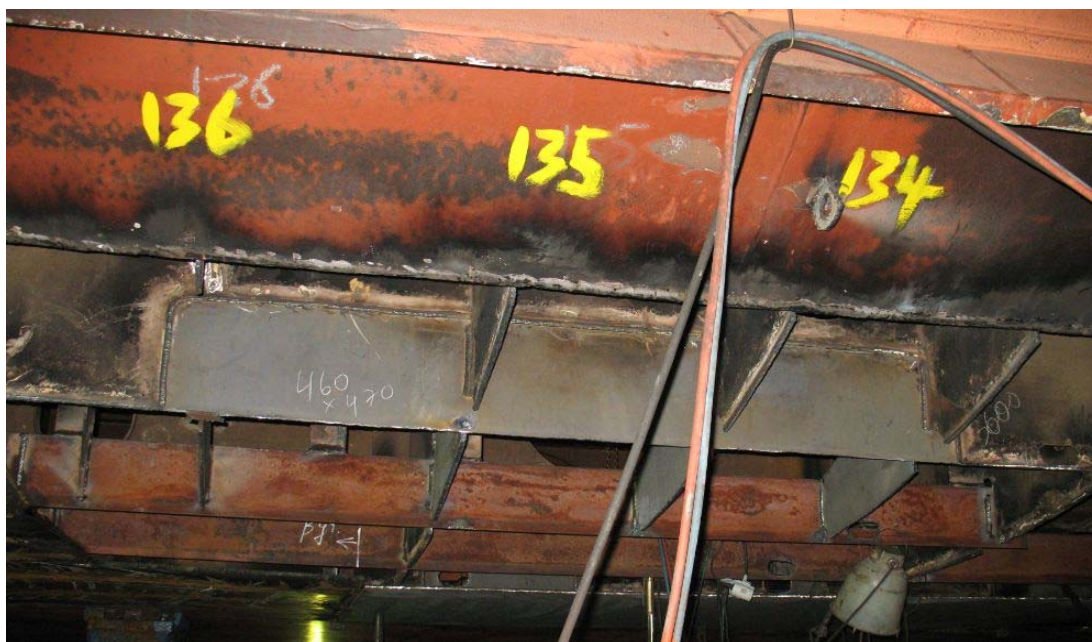
Figure 9. Damages to the vessel; a fixed tear in the port-side ballast tank.
