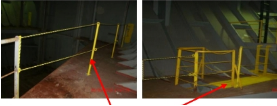
Figure 6. A Safety fence installed after the accident on the left and the painted passage on the right.
