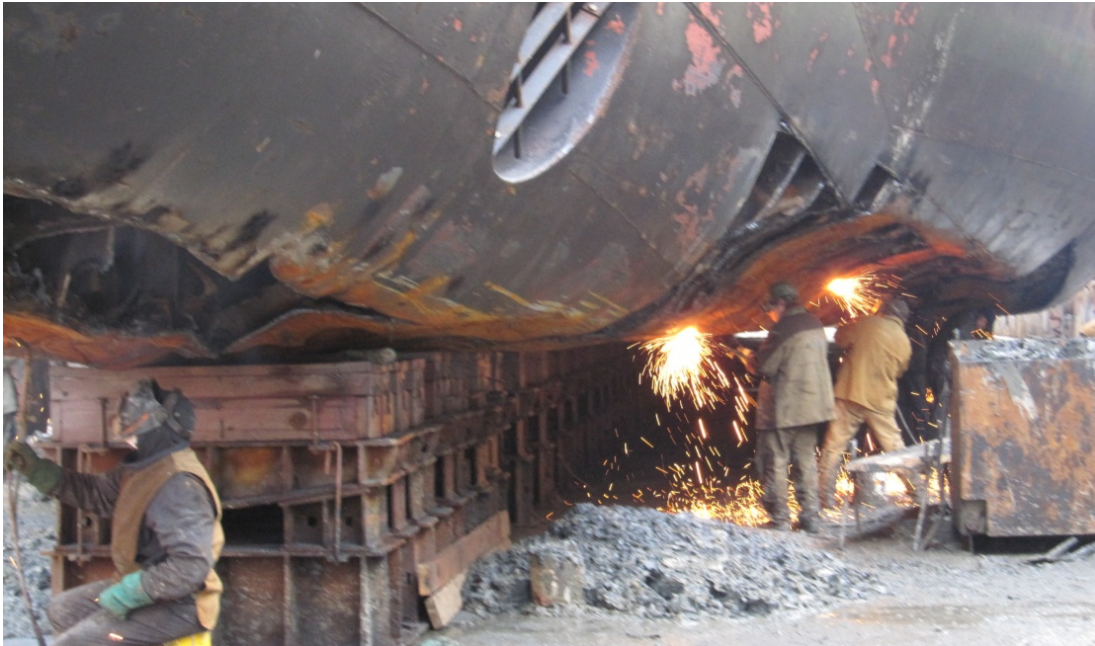
Figure 8. Damage to the port side of the bow.
