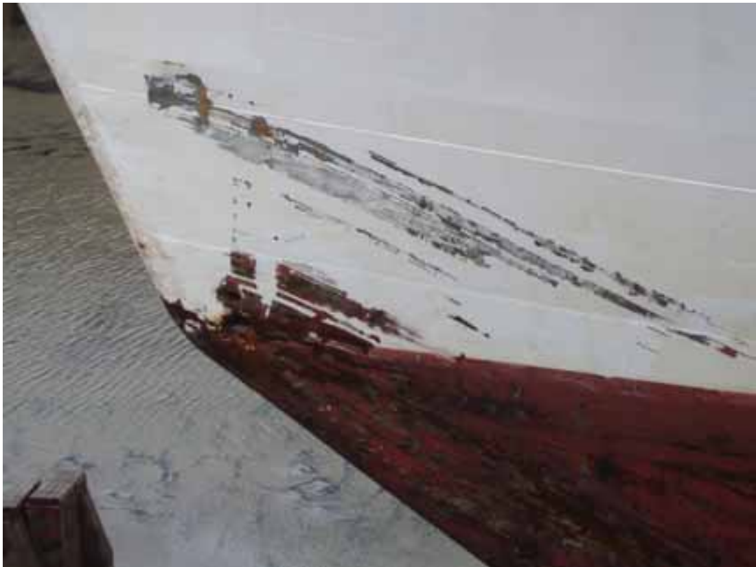
Figure 5. Damage to KRISTINA REGINA on the bb side
