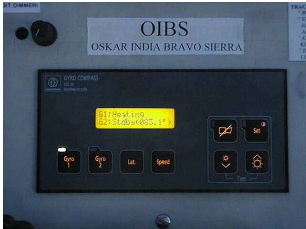
Figure 26. Gyro control panel on the FINNFELLOW. In the situation pictured here, the operative gyro is in the HEATING status and the second gyro (in stand-by status) shows the correct readings.
