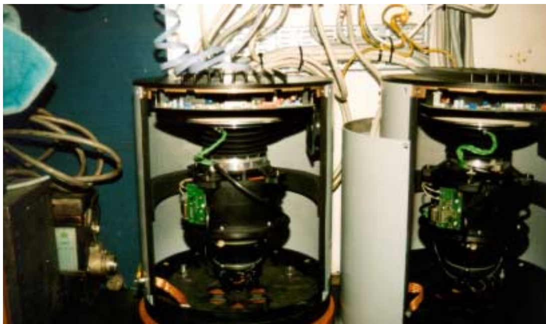
Figure 12. The Finnfellow's compass installation photographed during testing on the dock after the grounding. The coiled signal cable is visible behind gyrocompass number 1 on the left.
