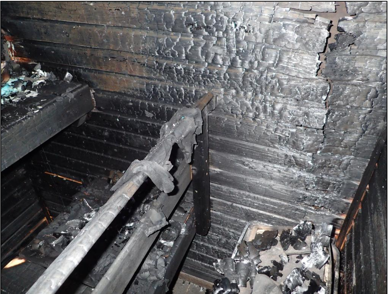
Kuva 1. There were clothes drying on the railings of the sauna stove and items were stored on the seats. The wall and ceiling panels in the sauna were charred during the fire and they partially burned through. (Photo: SIA)
