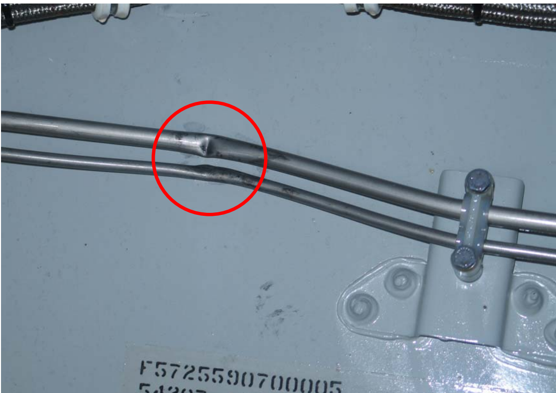
Figure 7. Damaged hydraulic lines
