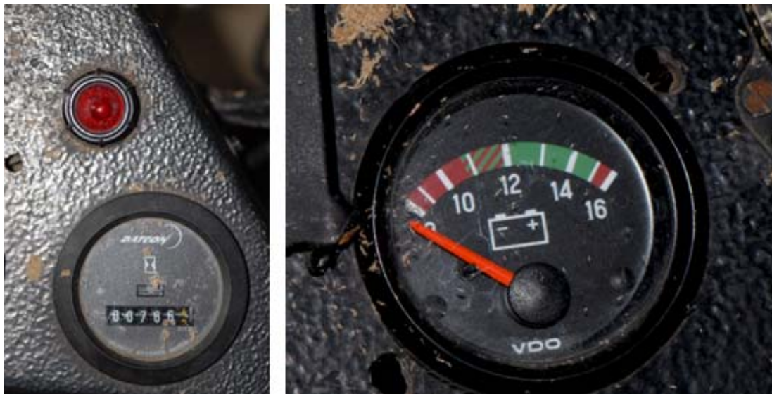
Figures 2 and 3. Generator warning light and Volt meter
